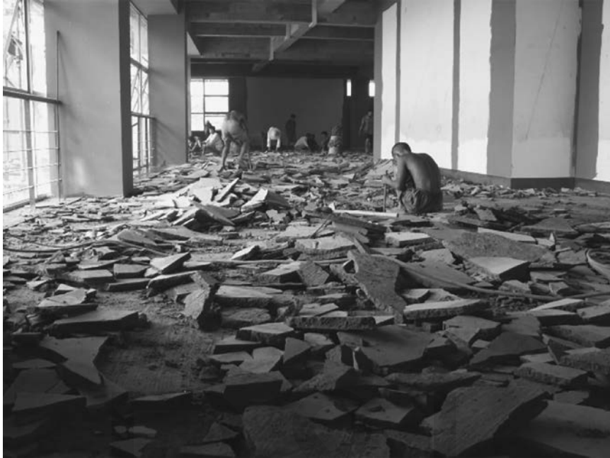
Figure 4.2. Builders working on the early JMC museums in 2005, courtesy of the Jianchuan Museum Complex
